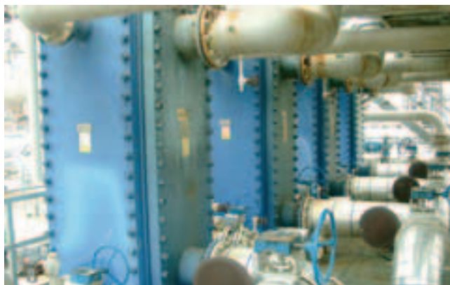
Four of the eight Compabloc condensers.
